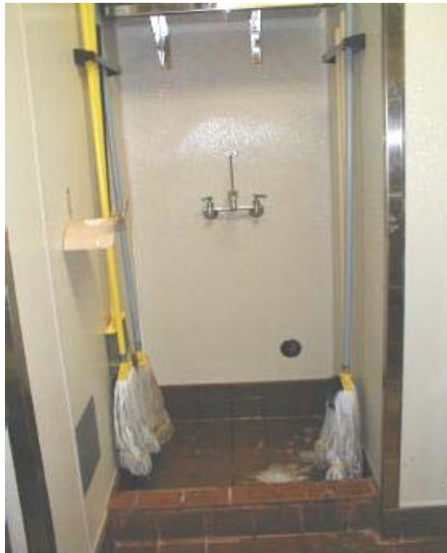
Figure 10 Janitorial Station With Slab Basin
